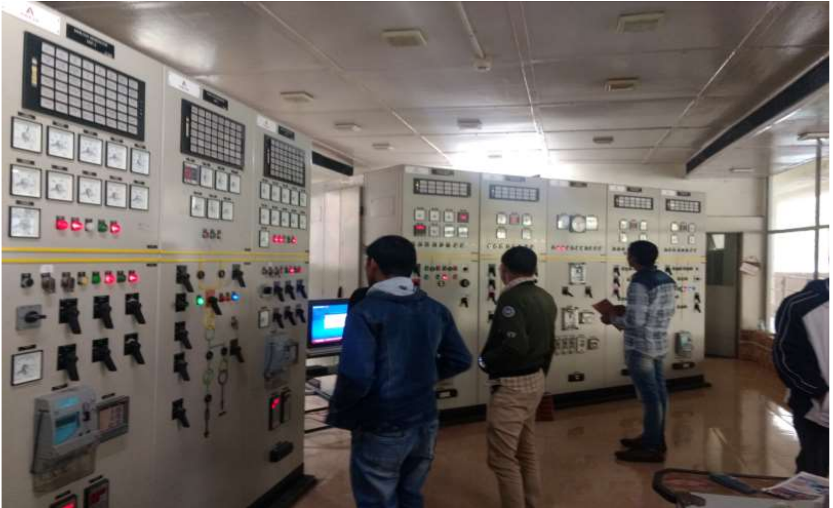
Figure of The Control Room of Umiam Power Station.
